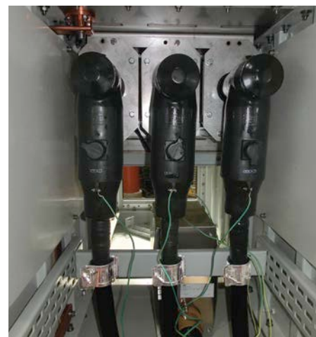
1250 A Cable Compartments
