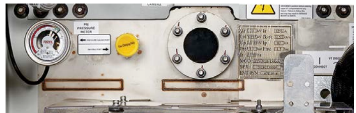
Tank View Port
