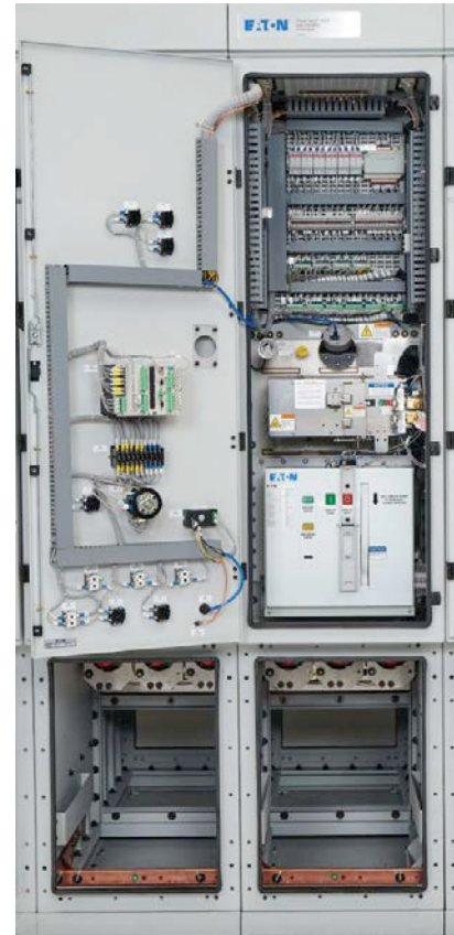
XGIS LV Compartment Door Open
