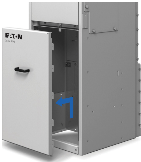
Figure 3-4: Opening the cable door for access
