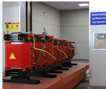
Partial discharge laboratory
